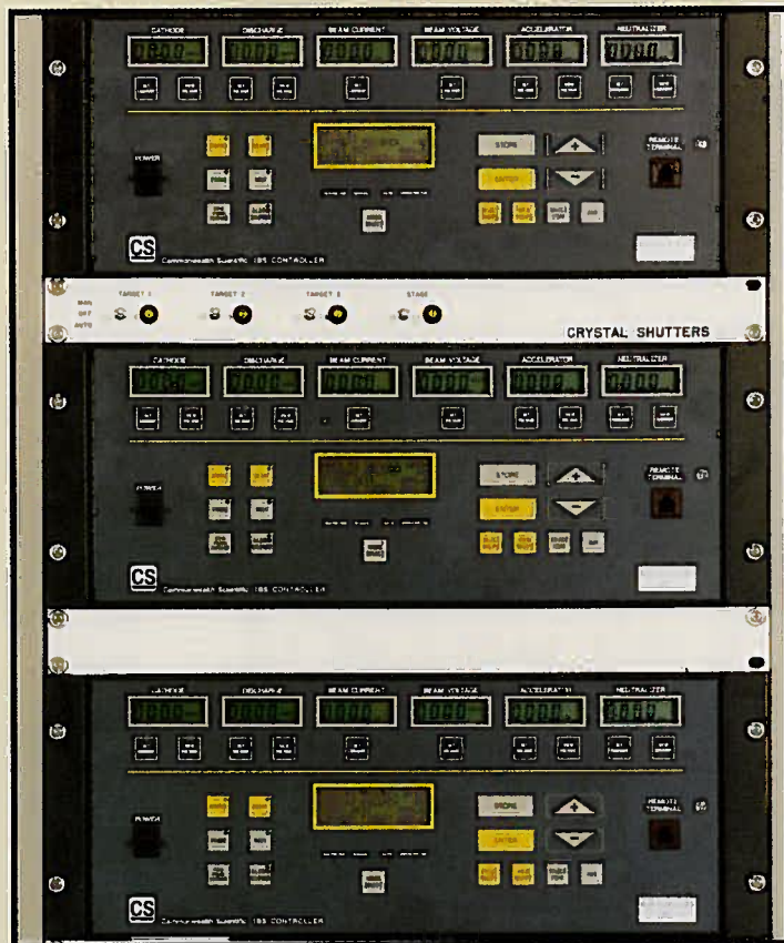
IBS Power Supply in system rack
